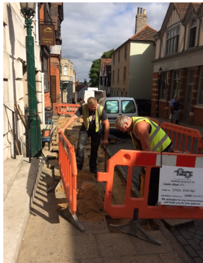
More than 5km of new duct, and 8km of fibre optic cables, were installed during the deployment of the Town Centre fibre optic network in 2016
