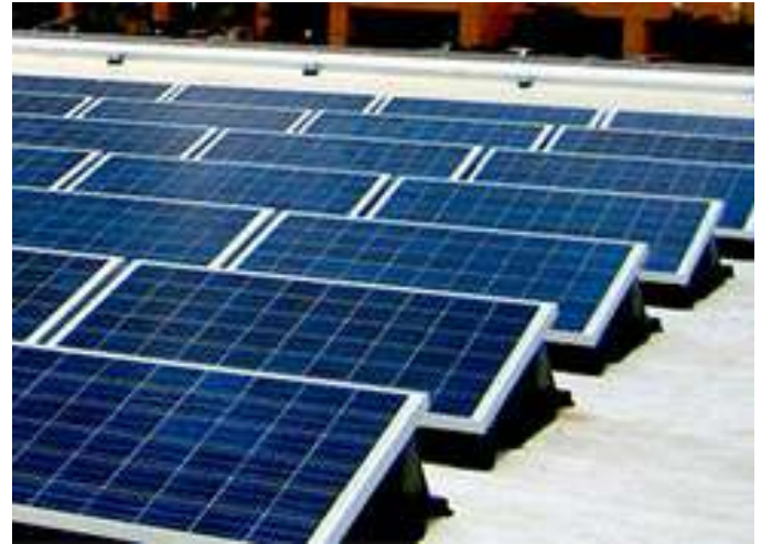
FIG 3.20.1. PHOTOVOLTAIC SOLAR PANELS.
