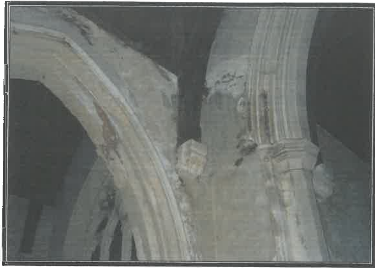
SIGNS OF DAMP AT WALL/ROOF
