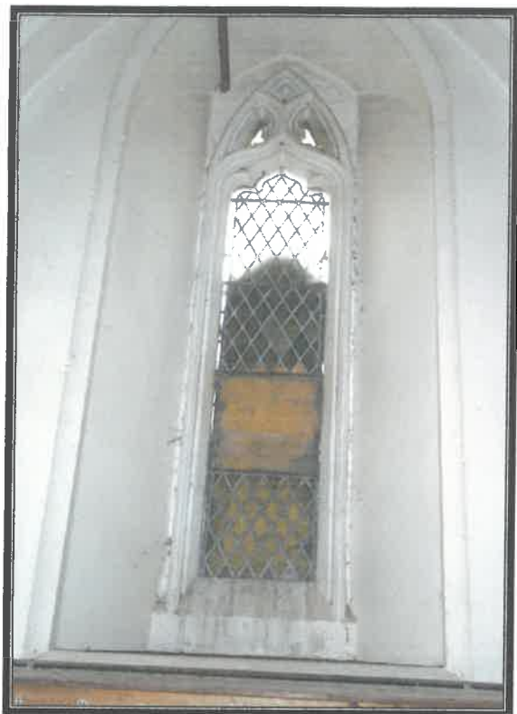
DAMAGED LEADED LIGHT WINDOW
