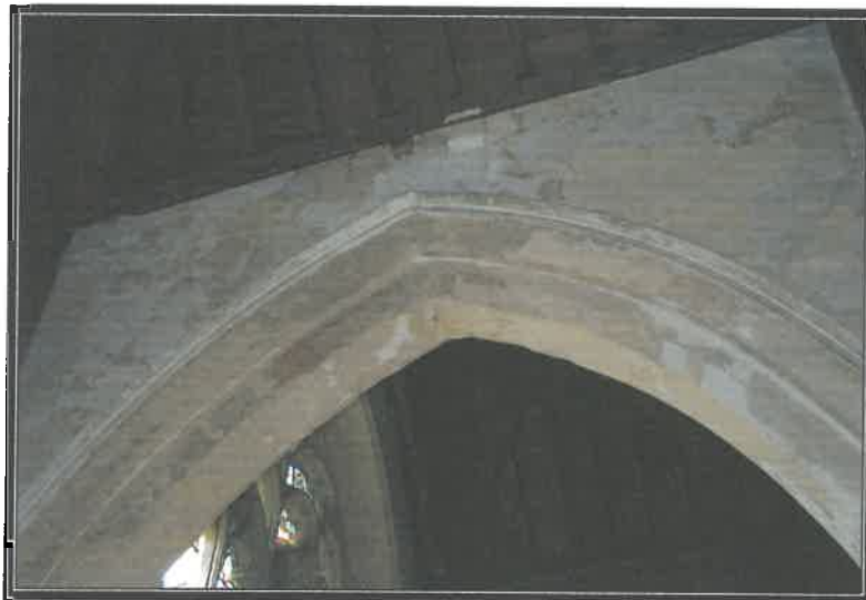
SIGNS OF DAMP AT WALL/ROOF
