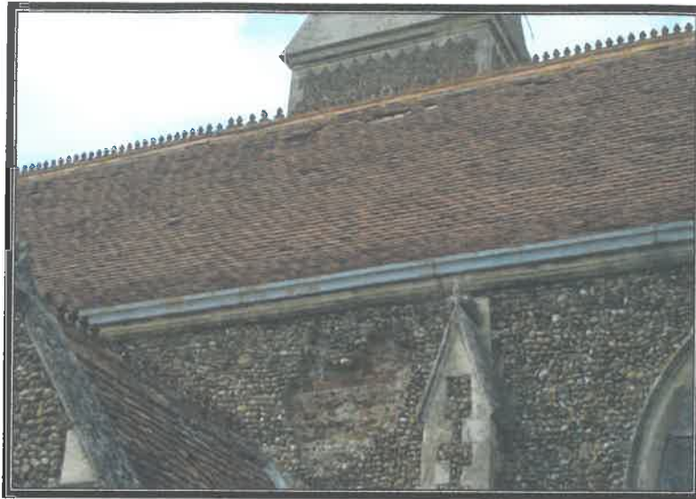
DEFECTIVE STONE FLINTS
