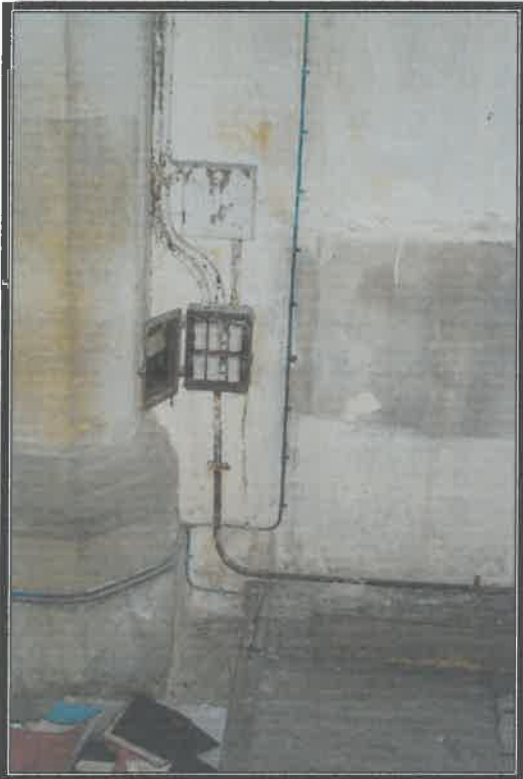
CORRODING FUSEBOX IN CHANCEL
