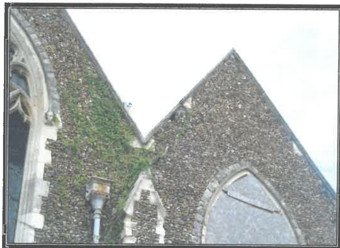
IVY GROWTH TO EXTERIOR AND MISSING STONWORK AT ENTRANCE
