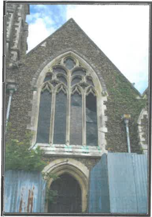
DAMAGED STAINED GLASS WINDOW AT ENTRANCE
