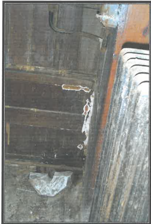
DAMP/FUNGAL GROWTH TO VESTRY
