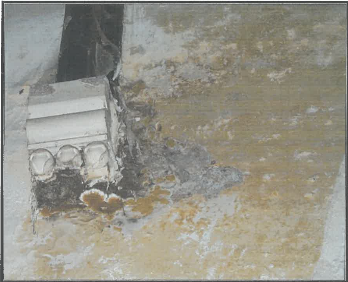
SIGNS OF DAMP AND FUNGAL GROWTH AT HIGH LEVEL CORBEL
