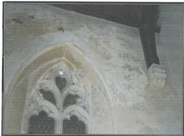
SIGNS OF DAMP AT WALL/ROOF
