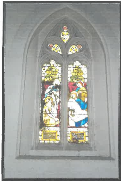
INTACT BUT UNPROTECTED STAINED GLASS WINDOW
