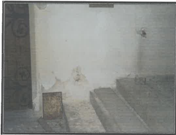
DAMAGED WALL IN CHANCEL
