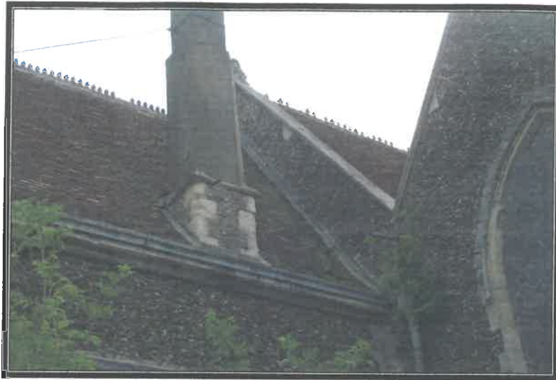
VIEW OF BLOCKED GUTTERS AND RAINWATER PIPE TO CHANCEL
