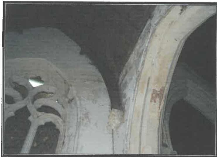
SIGNS OF DAMP AT WALL/ROOF
