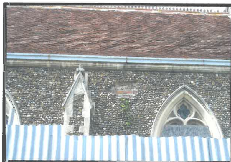
SECTION OF MISSING EXTERNAL STONE FLINTS TO RIGHT HAND SIDE OF CHURCH
