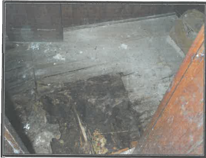
ROTTEN FLOOR TIMBERS TO VESTRY
