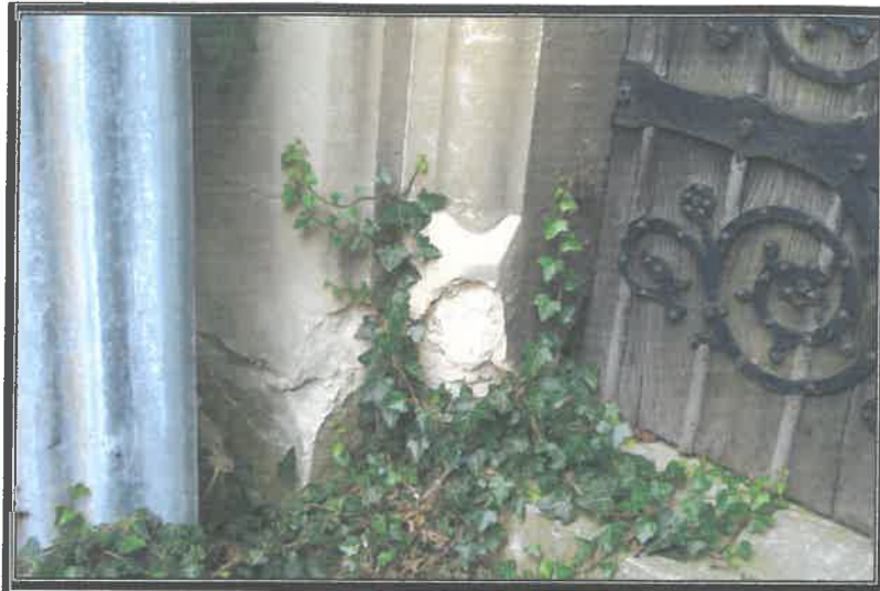
DAMAGED STONWORK TO FRONT ENTRANCE
