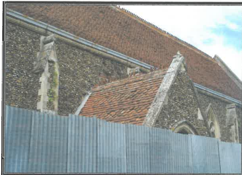
MISSING STONE FLINTS TO RENDER AND DAMAGED STONEMWORK TO RIGHT HAND SIDE
