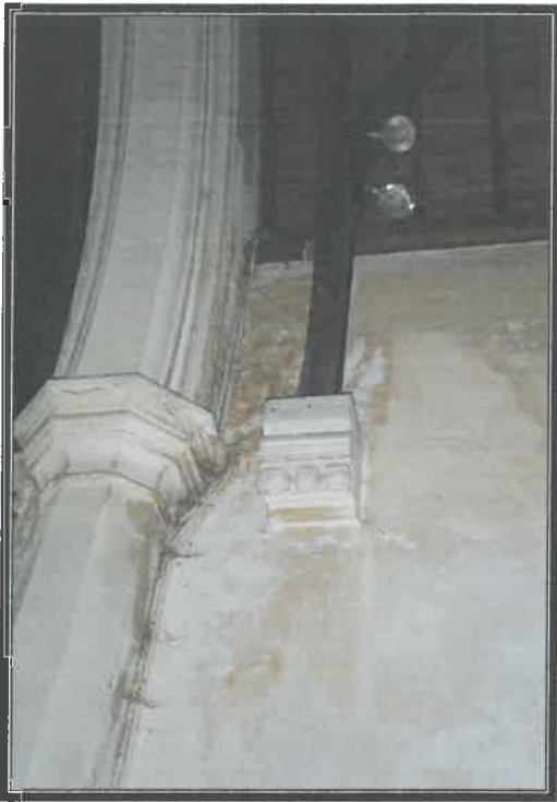
DAMP TO WALL IN CHANCEL
