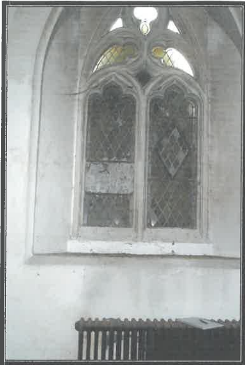
BROKEN GLASS TO BOARDED WINDOW
