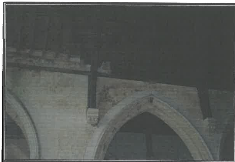
SIGNS OF DAMP AT WALL/ROOF
