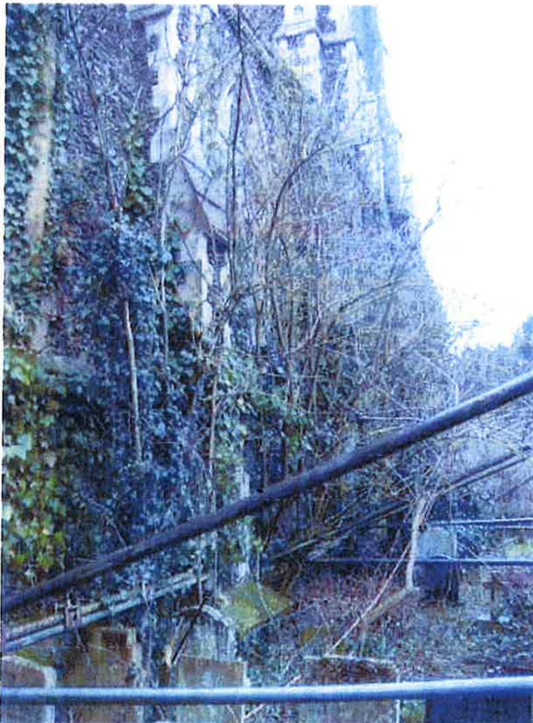
Image 06: Vegetation growth along the north elevation
