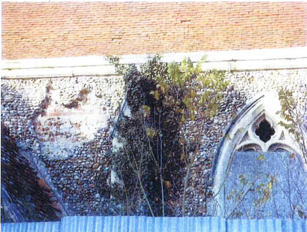
Image 03: Area of flint collapse above porch roof
