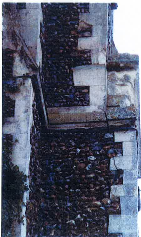
Image 07: Cracked masonry to the tower
