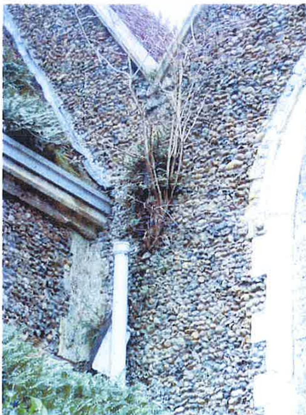
Image 05: Vegetation growth and damaged rainwater fittings
