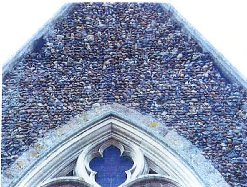
Image 04: Flint work falling away below copings
