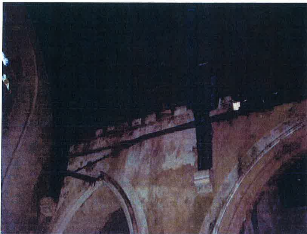
Image 12: Water penetration at high level to the nave, note daylight coming through
