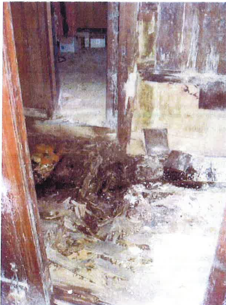
Image 11: Collapsed floor to cubicle vestry
